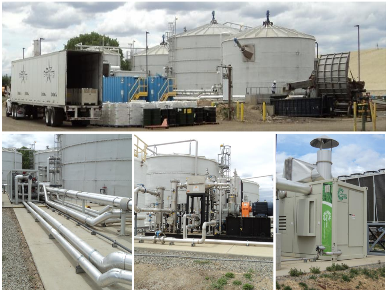
Figure C.4: CleanWorld HS-AD system schematic and UC, Davis facility photographs from field visit in May, 2015. Process schematic (top) (from Zhang, 2013) and UC, Davis facility view from the entrance (middle) and piping, pumps, and micro turbine set (bottom, left to right).
